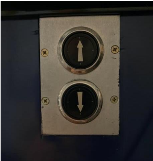
Fig. 78 Activation of drilling machine transport system B3, developed by A. van Ooyen.
